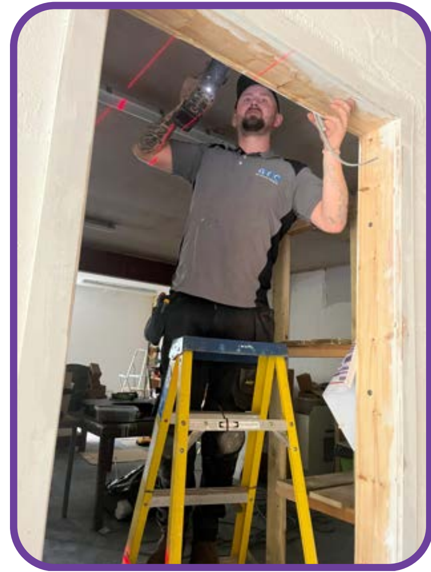
A huge thank you to George and Jason from GRG Projects, our excellent electricians, for brightening up our workshop with daylight strip lights, sockets and fire exits.
